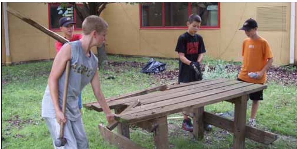
Youth from the Southern Illinois District made a great demolition team, clearing out old picnic tables that have outlived their usefulness in a courtyard that will serve as a playground at Unity Lutheran Christian Elementary School in East St. Louis.
